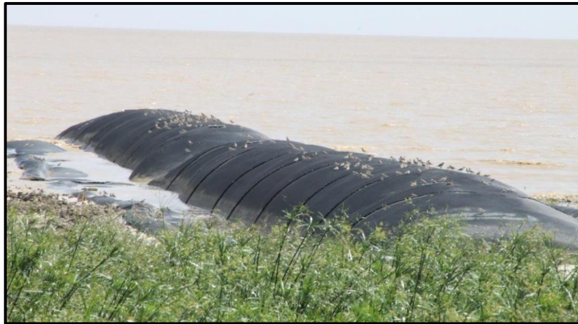
Figure 10: Completed 100m geotextile tube groyne, Reliance, Essequibo Coast, Region No. 2 during high tide. Date: 12 Dec 2017
